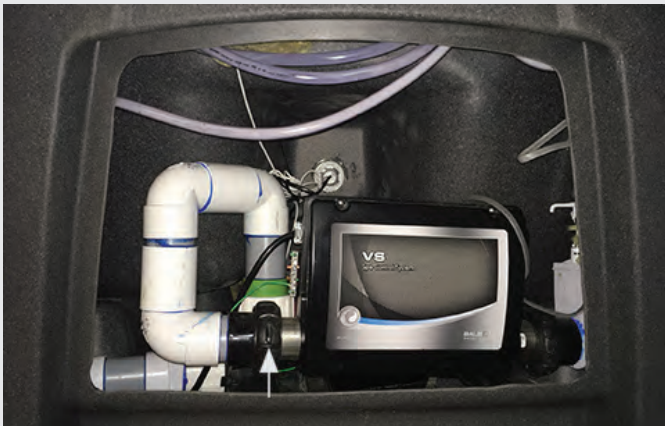
FIGURE 1.9a : HEATER UNION; LOOSEN UP TO BLEED AIR
